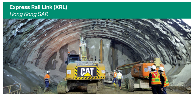
Largest rock cover (650 m) and longest tunnel (7.6 km) in Hong Kong SAR
